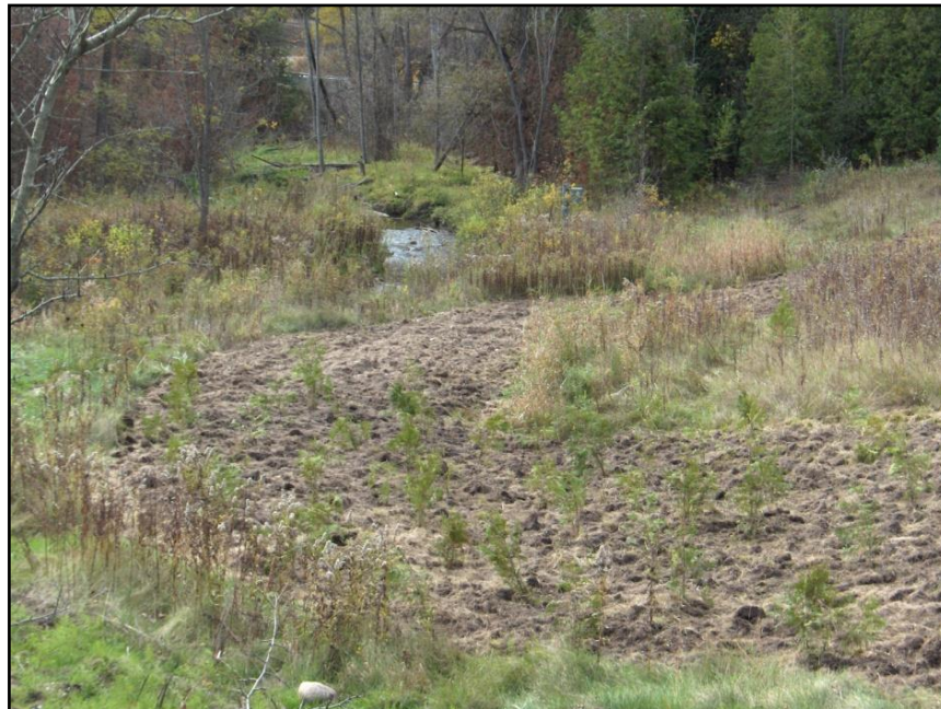
Figure 1: Photo taken after the restoration site was planted at the Claremont O.E.C, the creek where the gabion basket was removed is in the background.
