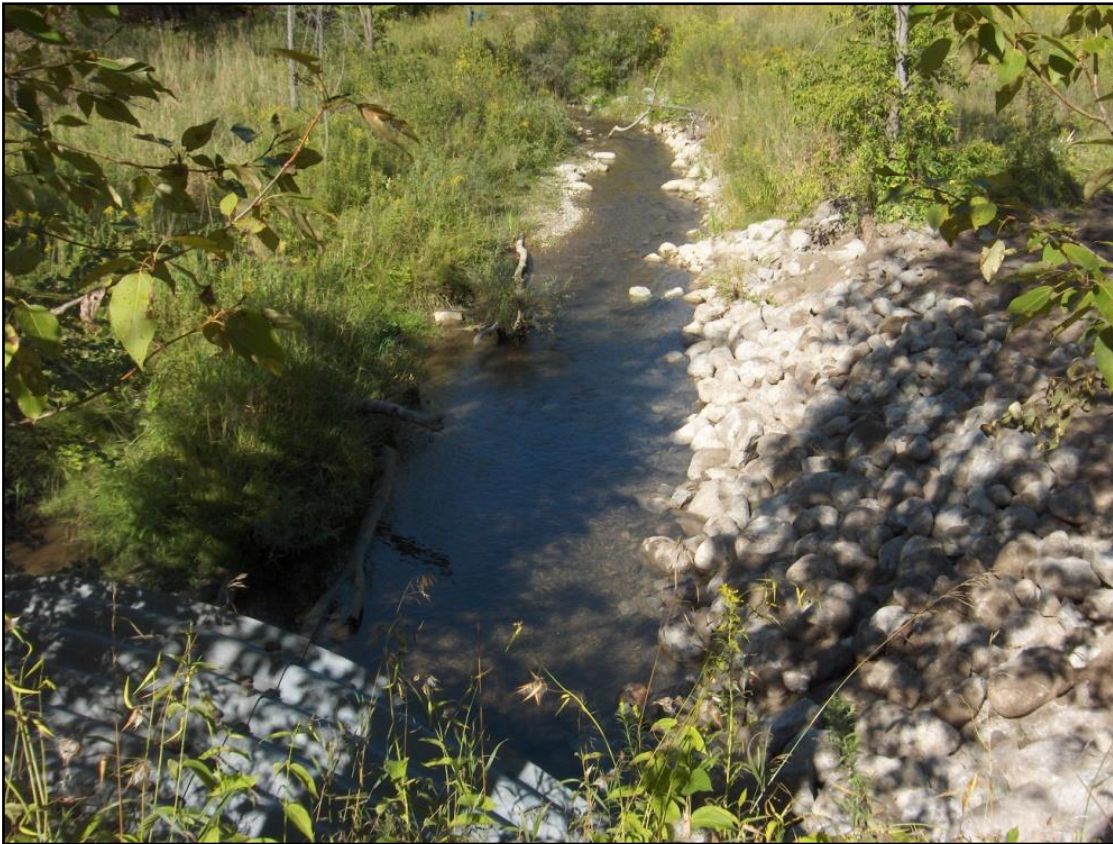
Figure 2: completed naturalized look of large boulders in replacement of the gabion basket.
