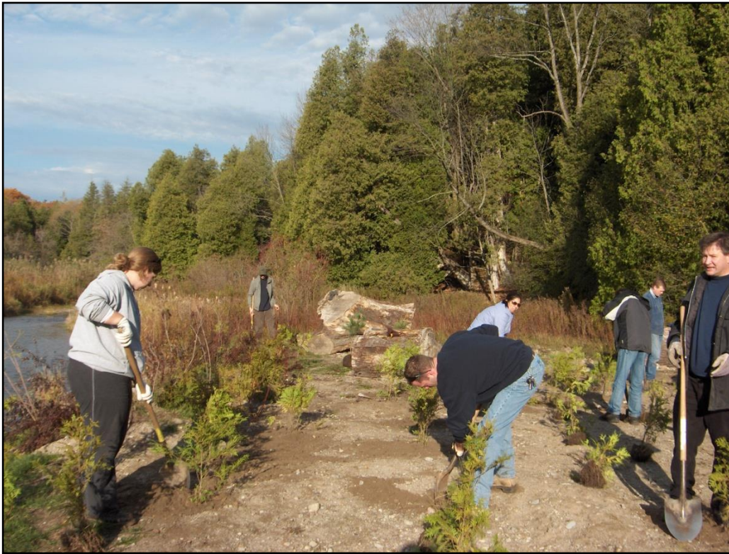
Figure 2: Community members volunteer their time to plant white cedars next to the newly constructed live cribwall at the Greenwood Conservation Area.
