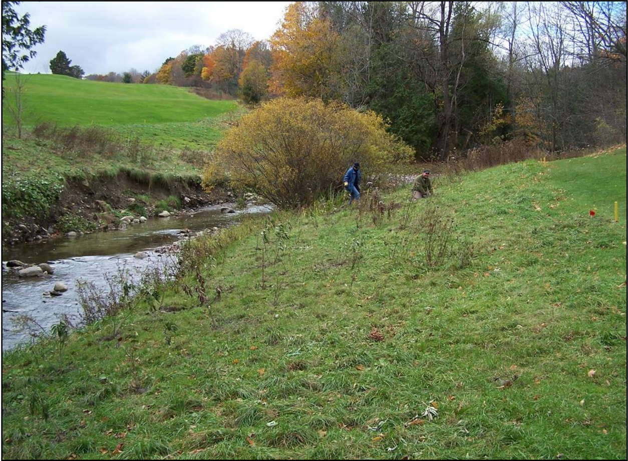
Figure 2: Shoreline at Golf Course being planted with live bare root shrubs in the fall of 2008.
