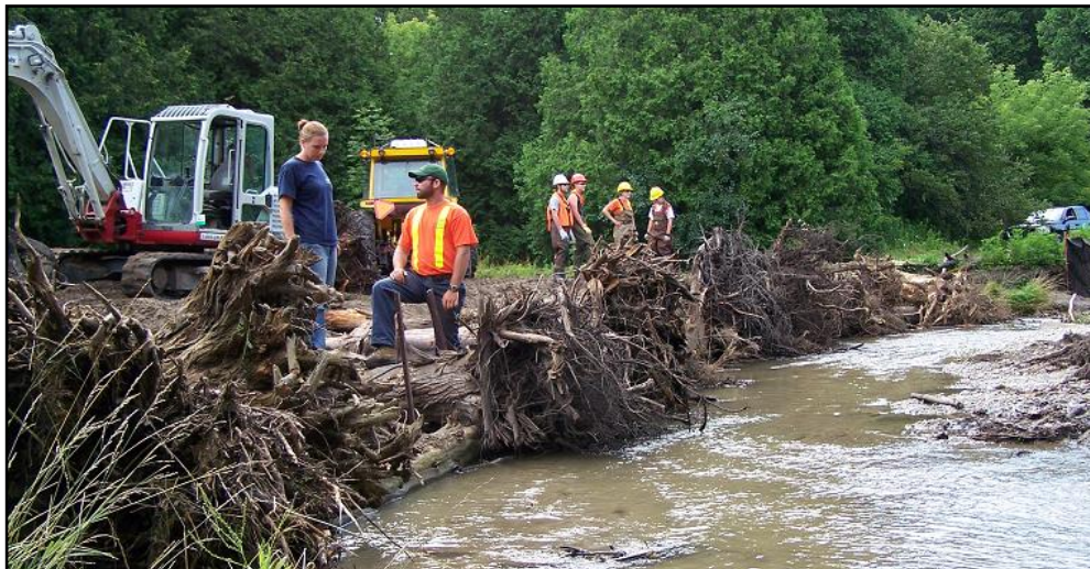
Figure 1: Root wads and woody debris being placed along stream bank to stabilize the shoreline.
