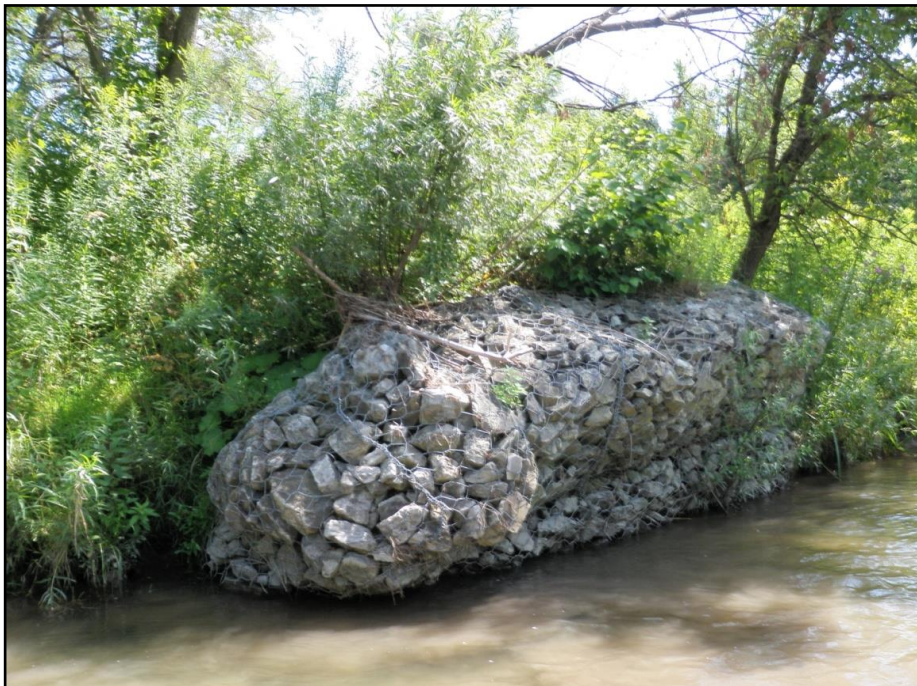
Figure 1: Failing gabion basket along Duffins Creek in Greenwood Conservation Area.
