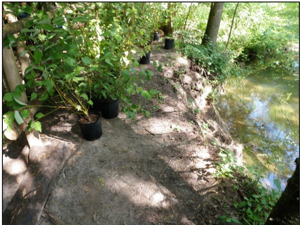
Figure 1: Image of unstable stream bank along Cobourg Brook at the Laurie Lawson Outdoor Education Centre.
