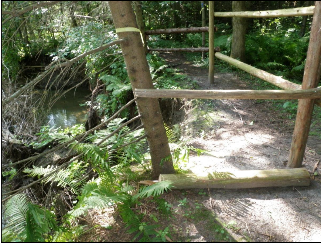
Figure 2: Fencing put in place along the bank to keep trail users back from failing slope and to protect newly planted dogwood shrubs.
