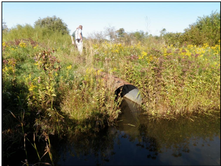
Figure 1: Degrading culvert on Transport Canada Pickering Lands planned before removal.
