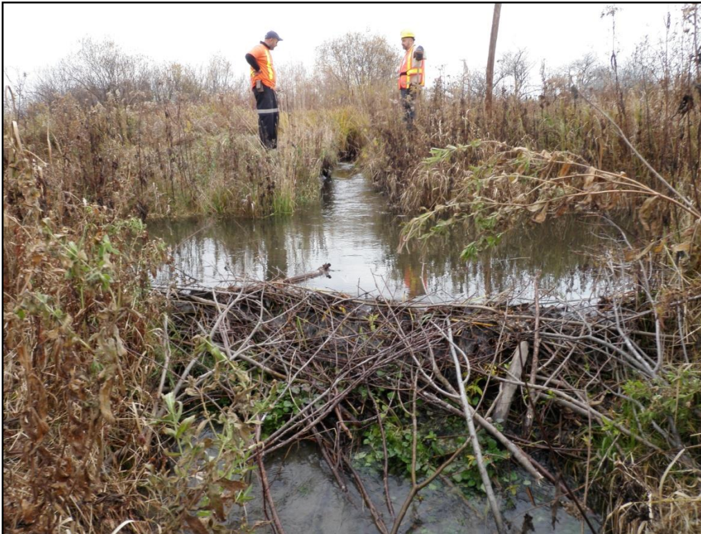
Figure 3: TRCA staff observing the removed culvert location, which appears to be in good condition.
