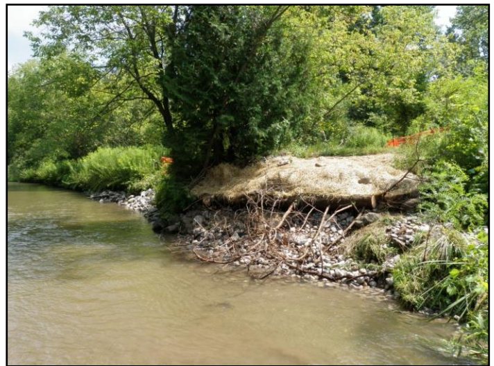
Figure 5: Completed footbridge removal and bank stabilization in Greenwood Conservation Area on Duffins Creek.
