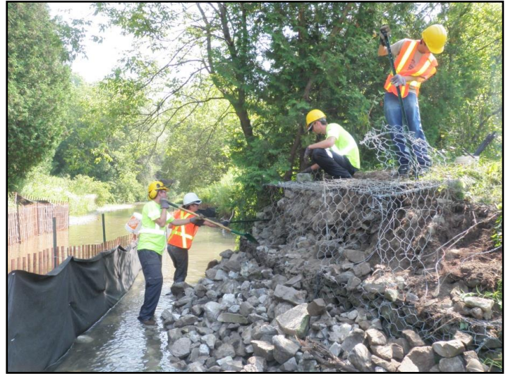
Figure 3: TRCA and OFAH staff disassembling stone gabions on either side of former footbridge.
