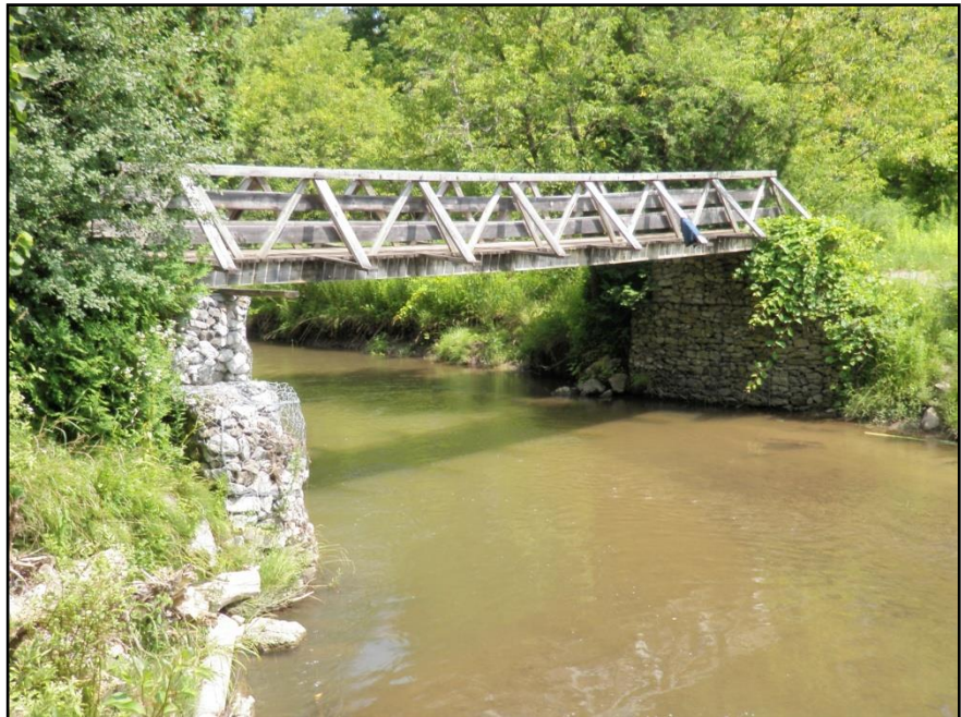
Figure 1: Failed footbridge in Greenwood Conservation Area.
