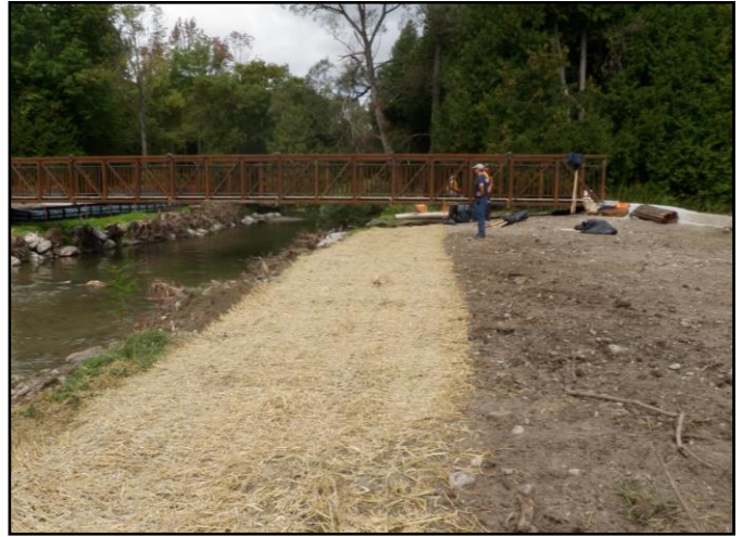
Figure 3: New bridge built and root wad and straw in place along banks of Duffins Creek.
