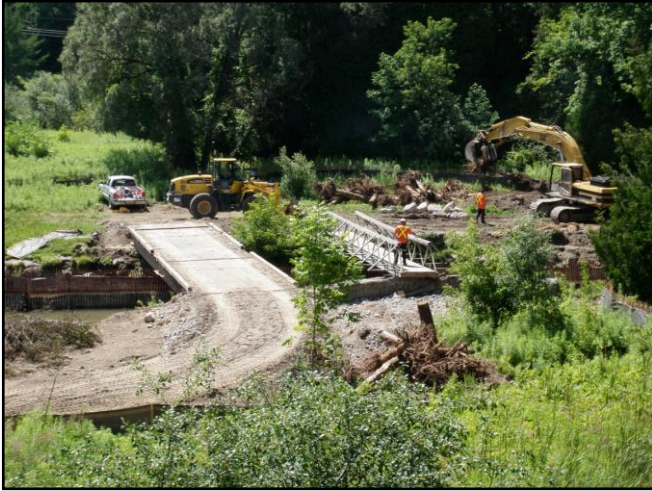
Figure 2: Building of new bridge and then dismantling of the old bridge will begin.
