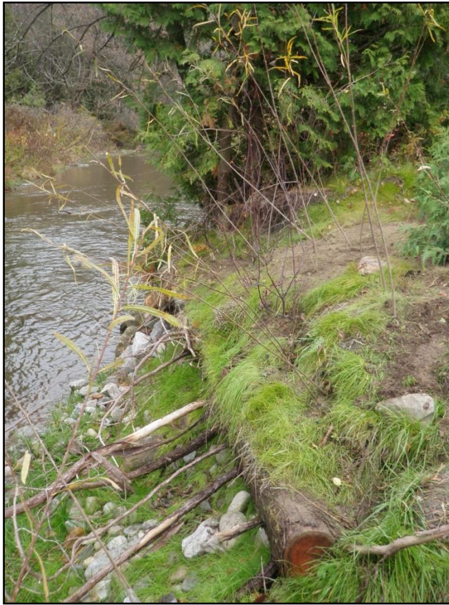
Figure 2: Live stake willows planted along bank, logs used for bank stability can be seen in the photo as well.
