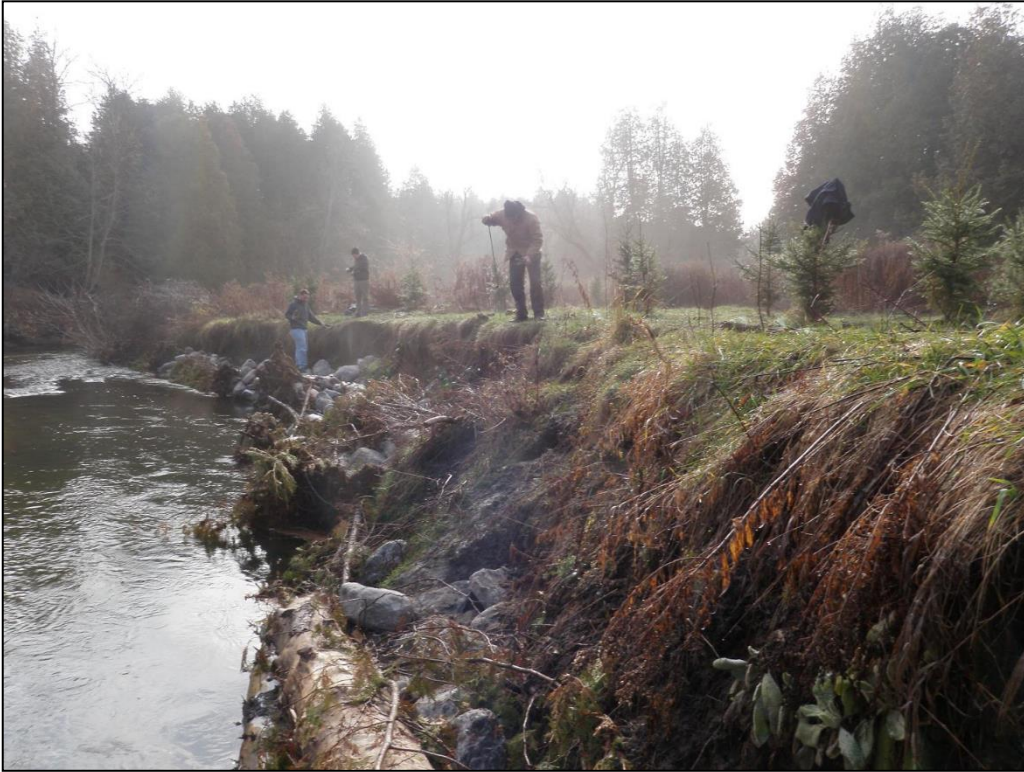
Figure 2: Live willow stakes being installed by TRCA, MNRF and a local volunteer.
