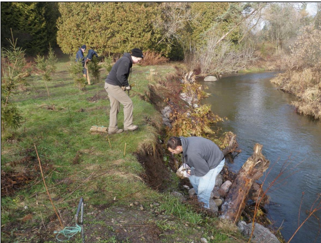
Figure 3: The crew inserting the live willow stakes on the lower and upper bank.
