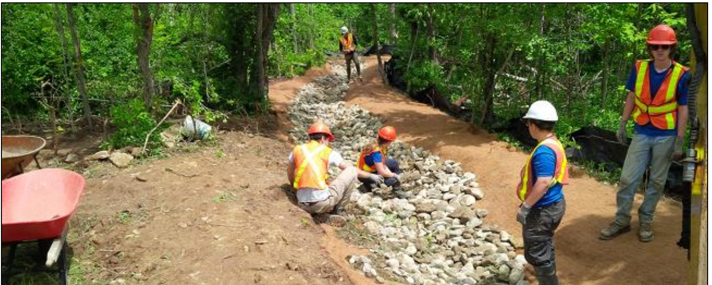
Figure 1: Ontario Streams workers installing the round river stone in the bottom of the bypass channel.
