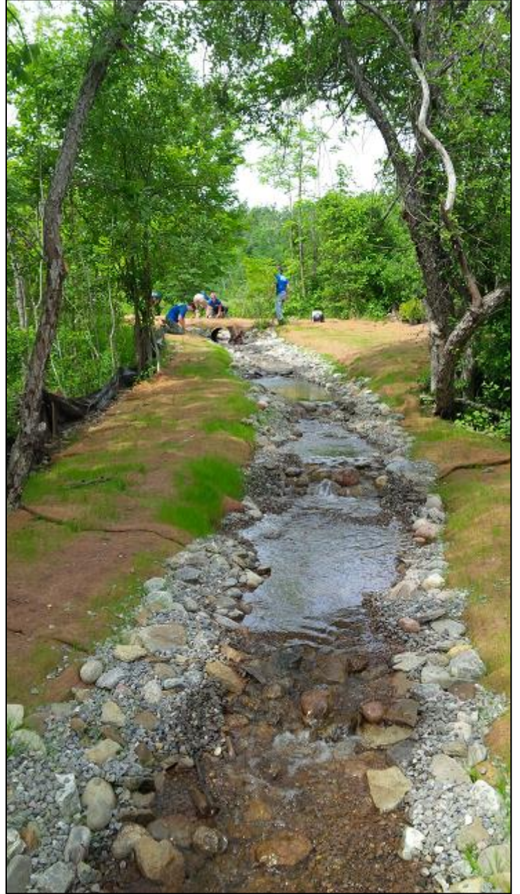
Figure 3: Bypass channel completed with water flowing, photo facing upstream towards the new culvert.
